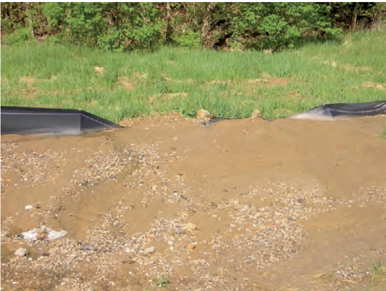
Plate 43 Sediment accumulation above silt fences can overtop them under concentrated flow erosion (Courtesy C.J. Gantzer Univ. of Missouri)
