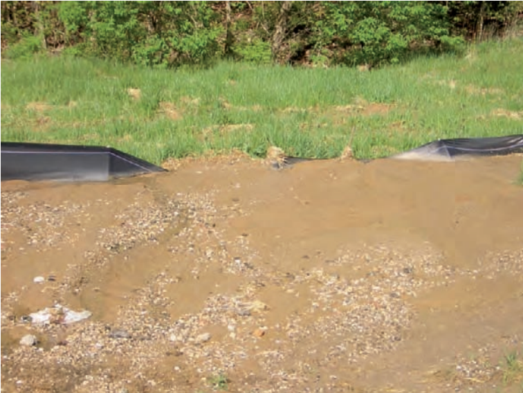
Fig. 11.1 Sediment accumulation above silt fences can overtop them under concentrated flow erosion (Courtesy C.J. Gantzer, Univ. of Missouri, Columbia, MO)
